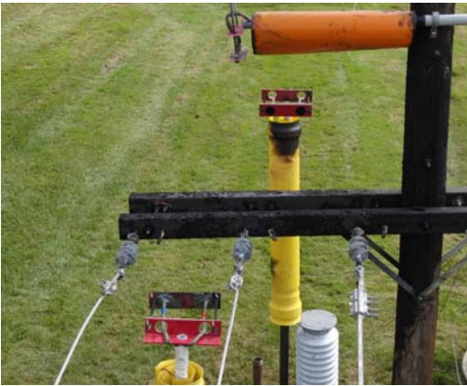
Fig. 9. Three-phase dead-end structure prior to an arc flash test.
