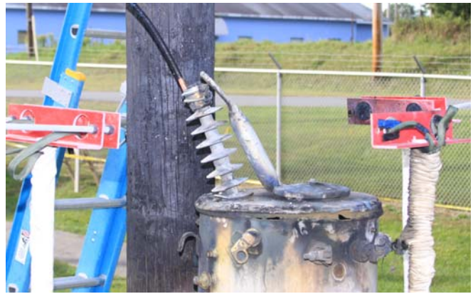
Fig. 2. Mock tool across the transformer bushing prior to a test.
