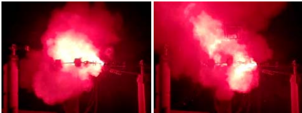
Fig. 10. Side view of a three-phase fault on a dead-end structure.
