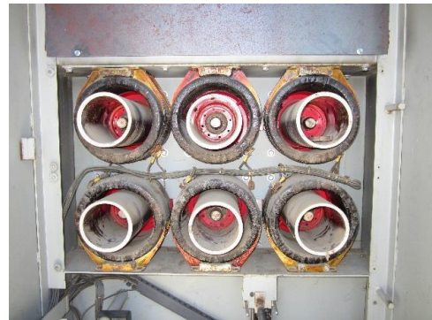
Fig. 11. Horizontal, rack-in-style stabs with the shutter removed.
